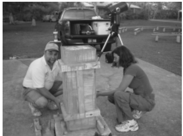
Nick and Vickie Van Ryn get ready to remove the wooden form around the concrete telescope mount.
