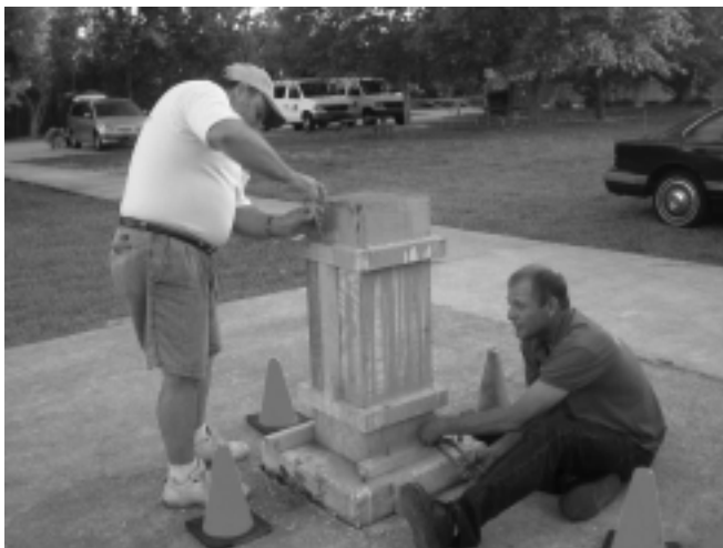
After pouring the cement into the wooden form, Nick measures accurately for the return of the SCAS metal plaque as Steve adjusts the form to due north.
