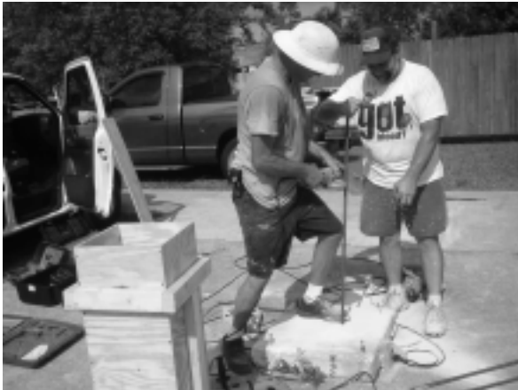
Steve Van Ryn (L) and Nick Stingone (R) measure rebar for the base of the mount.
